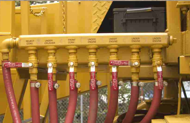
Dust Suppression - Seven Misting Spray Bars
